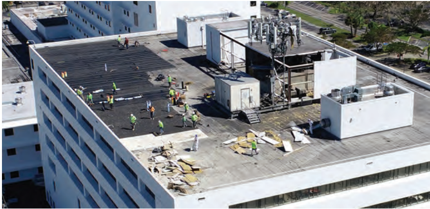
Roofing damage during Hurricane Ian was limited to those facilities, like Lee Memorial Hospital pictured here, where Lee Health had already scheduled roof replacements for later this year.
