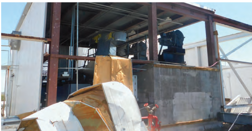
Damage to the elevator room in the medical office building housing Lee Health's rehabilitation hospital disabled the bank of elevators and required $1 million in repairs.
